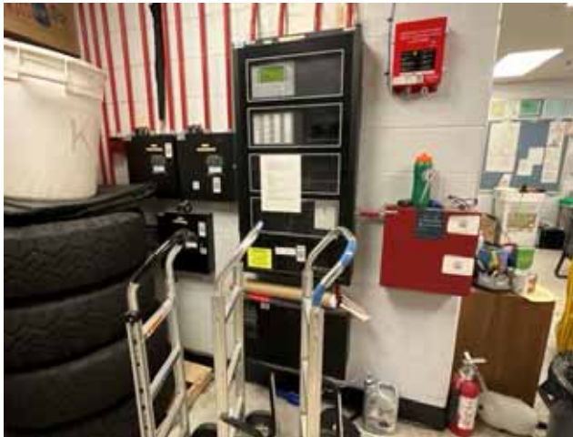
27 - FIRE ALARM PANEL
